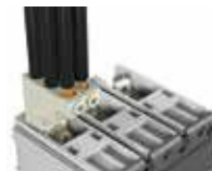
Multi-cable terminals with cables
