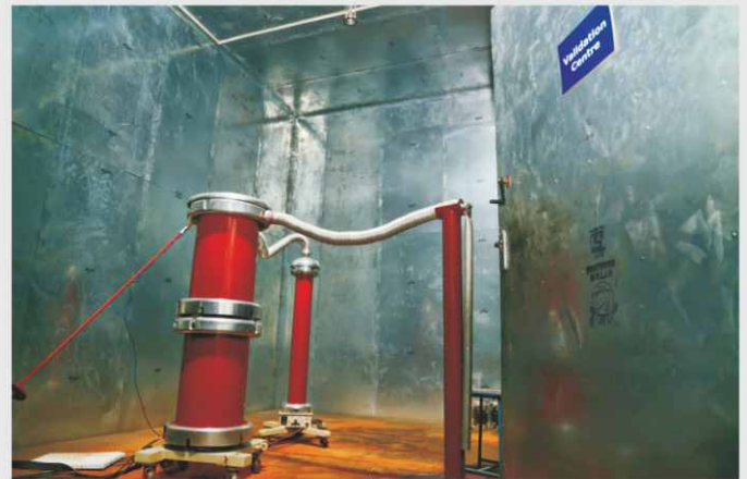
Partial Discharge Test
