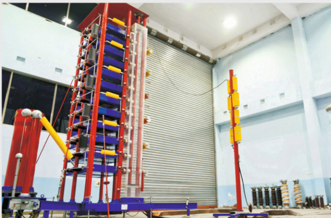
1200 Kv Impulse Voltage Generator
